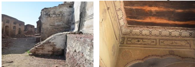
Figure 17 Decaying in building sue to long flooding of water (Source:Author)
